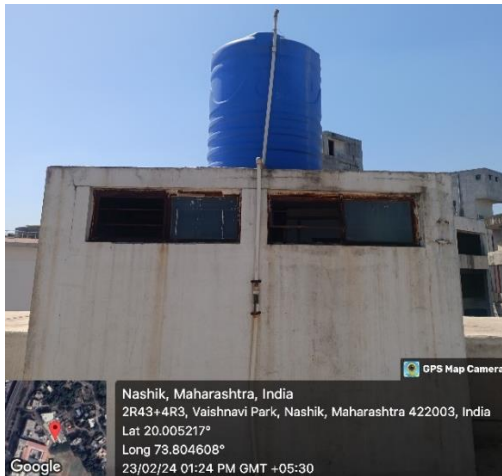
Overhead Water Tank – Girl’s Hostel
